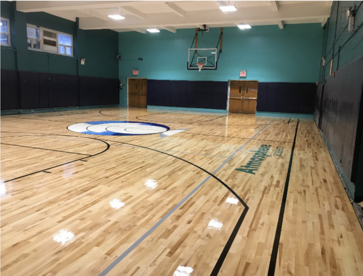
A brand new Connor Sports floor in the Riverdale School basketball court, installed by RD Weis Companies!
